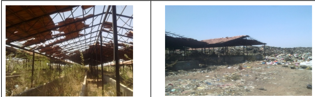
Picture 9 : VCP not being utilised and encircled with unsegregated solid waste at Surendranagar NP, Surendranagar District (22/05/2013)
